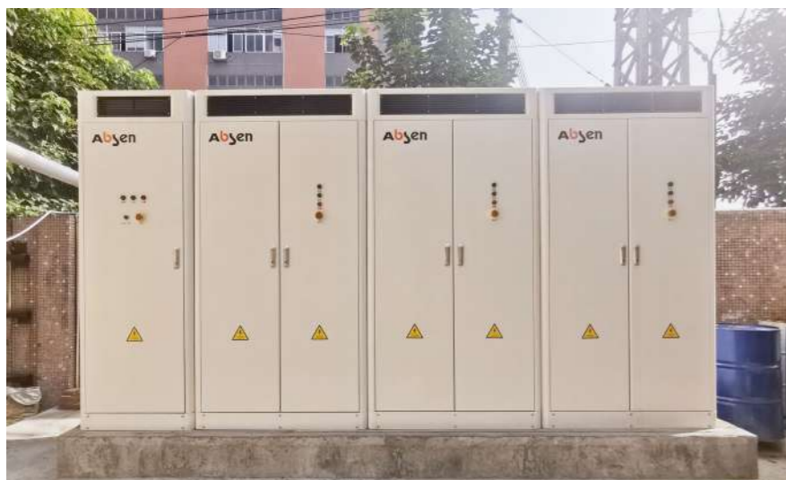
1.86MW/3.72MWh Zhongshan, Guangdong
