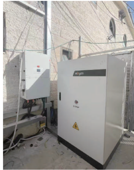
50kW/125kWh Middel East
