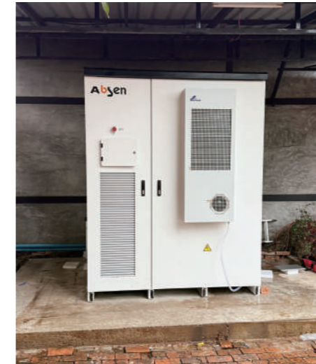
100kW/215kWh Myanmar, Mawlamyine
