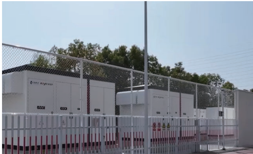
8.18MW/16.37MWh Suzhou, China
