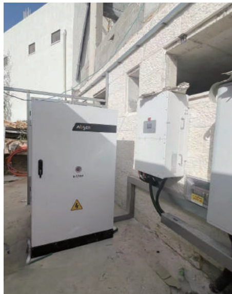
50kW/60kWh Middel East
