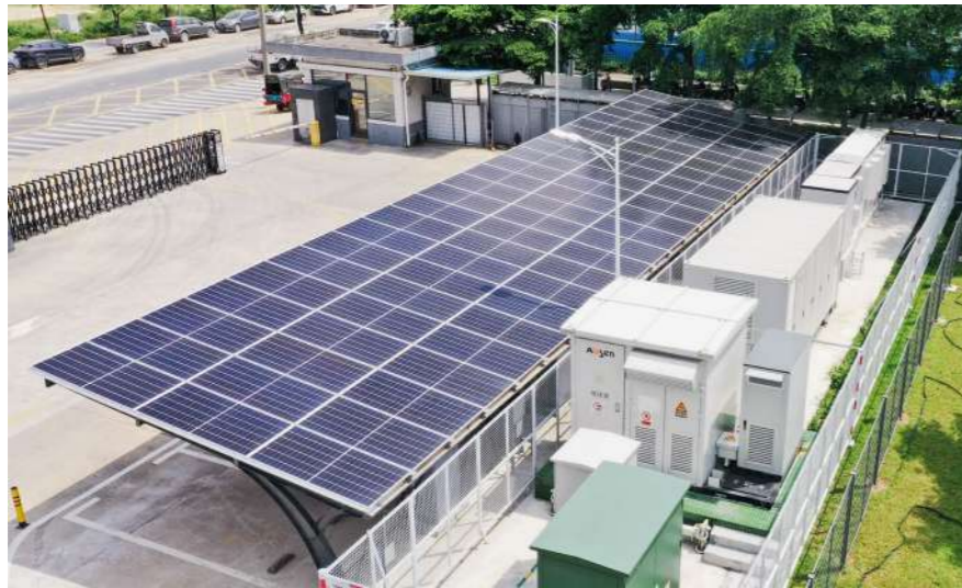
2.3MW/4.6MWh Huizhou, Guangdong
