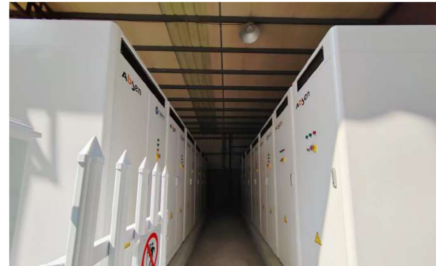
1.1MW/2.2MWh Dongguan, Guangdong
