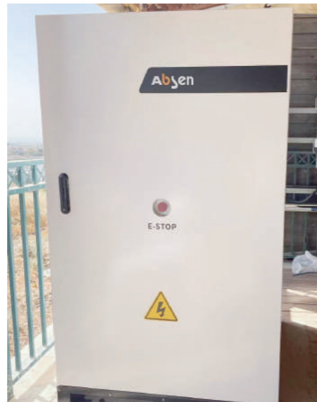
50kW/125kWh Middel East
