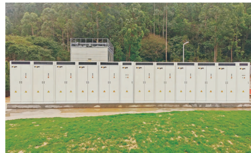
1MW/2MWh Huizhou, Guangdong
