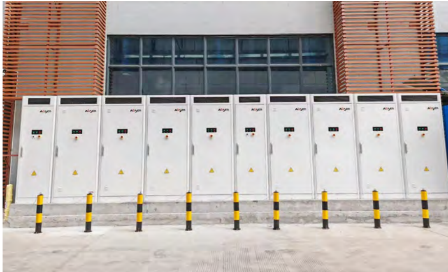
0.92MW/1.92MWh Guangdong, China
