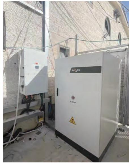
50kW/125kWh Middel East
