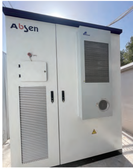
100kW/215kWh Middel East
