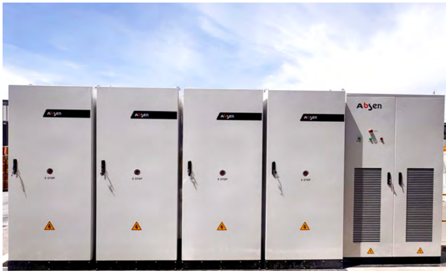
500kW/900kWh Arequipa, Peru
