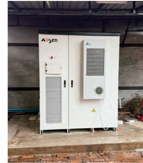
100kW/215kWh Myanmar, Mawlamyine
