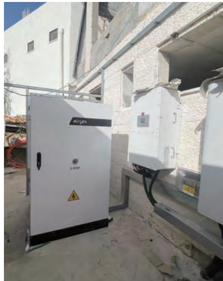
50kW/60kWh Middel East
