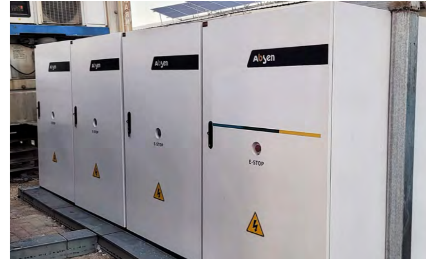
400kW/1024kWh Middel East
