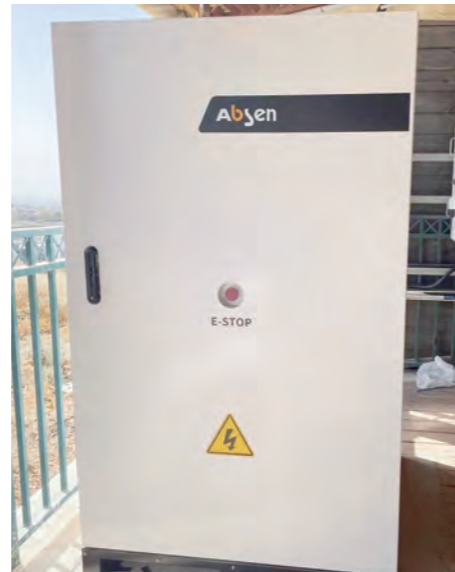
50kW/125kWh Middel East
