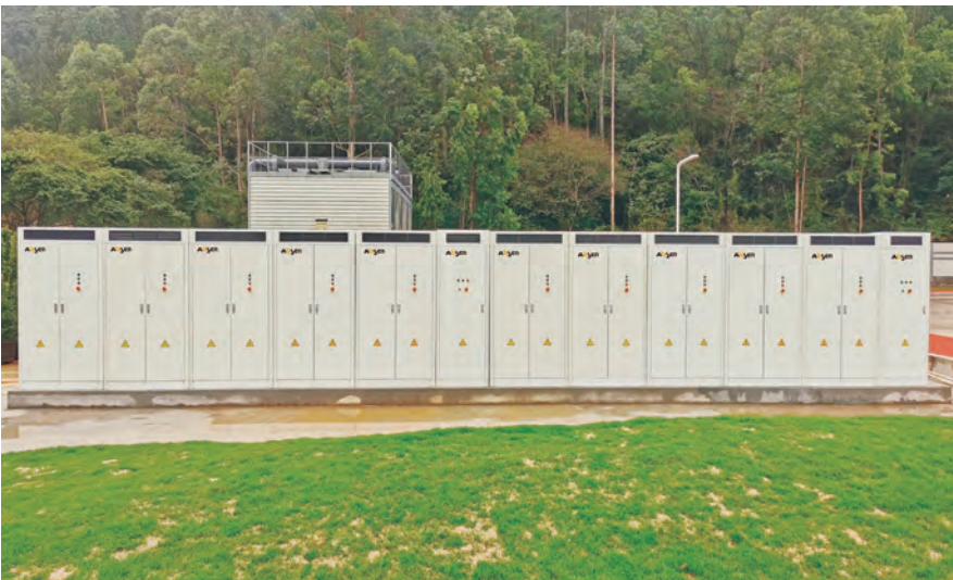
1MW/2MWh Huizhou, Guangdong
