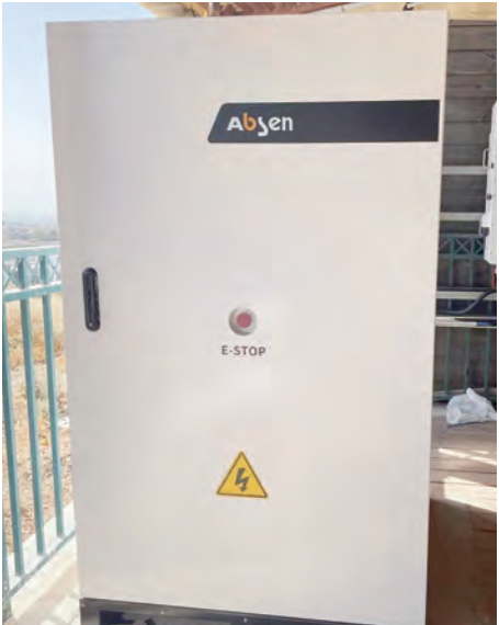
50kW/128kWh Middel East
