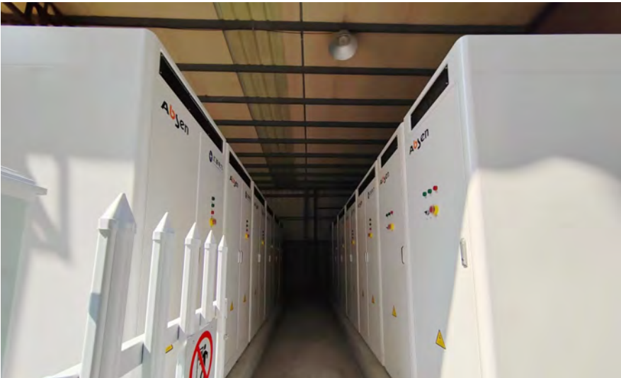
1.1MW/2.2MWh Dongguan, Guangdong
