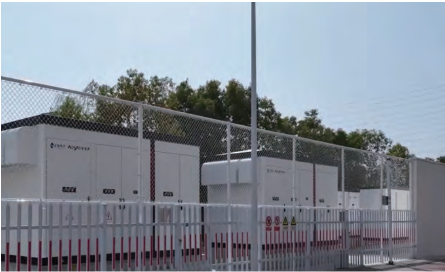
8.18MW/16.37MWh Suzhou, China
