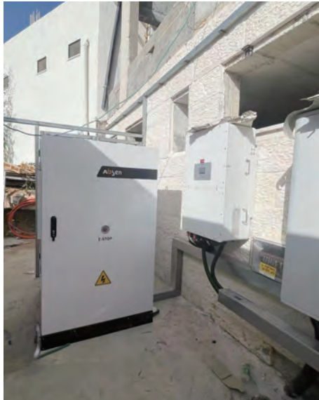
50kW/128kWh Middel East
