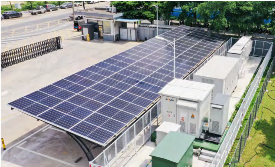
2.3MW/4.6MWh Huizhou, Guangdong
