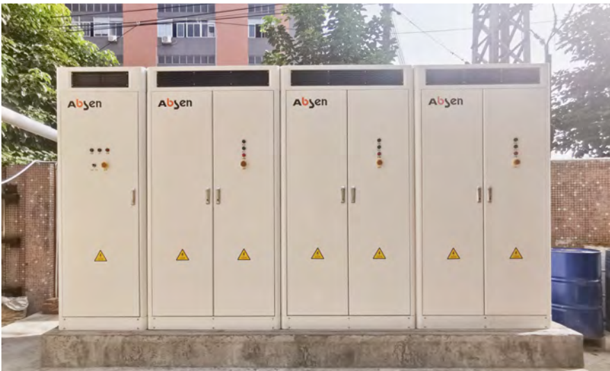
1.86MW/3.72MWh Zhongshan, Guangdong
