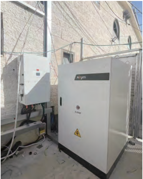
50kW/128kWh Middel East
